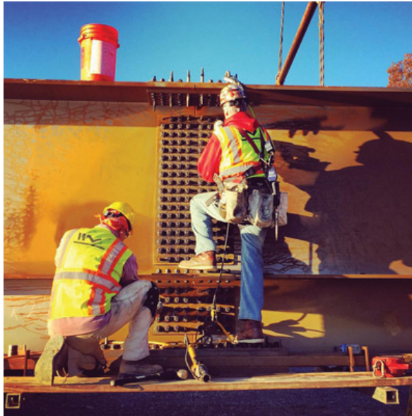
A sharp focus and precise workmanship, such as that demonstrated by these workers installing a girder splice, is critical to maintaining the public trust in delivering the Nation's highway program.
