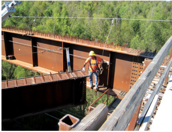
Proper construction techniques, such as the girder setting shown here, require specialized skill sets for the transportation workforce.
