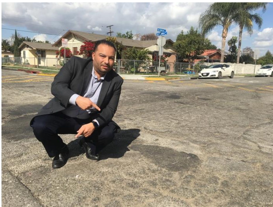
Lynwood Mayor Jose Luis Salache on deteriorated Duncan Avenue whose repair is accelerated with money from SB1, California's new gas tax.
